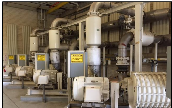
Multi-stage centrifugal blowers produce process air at the SEWRF.
