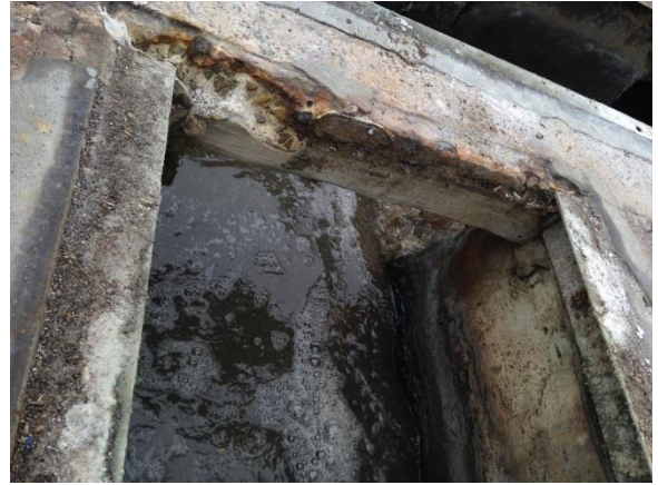
Grit Influent Channel
