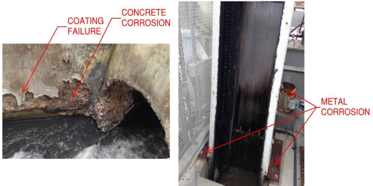
Figure 1. Equipment and Concrete Deficiencies
