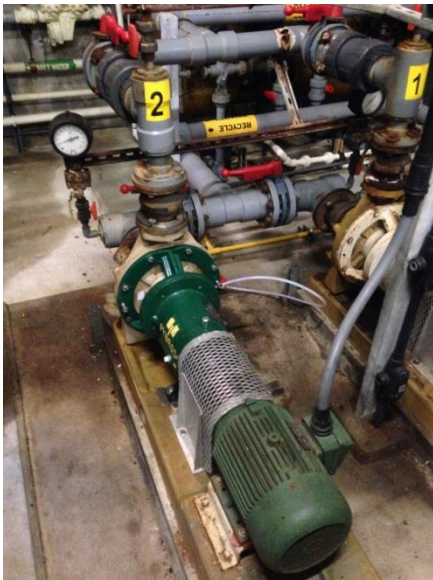
Chemical Recirculation Pump
