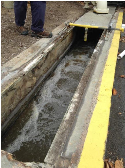
Grit Influent Channel
