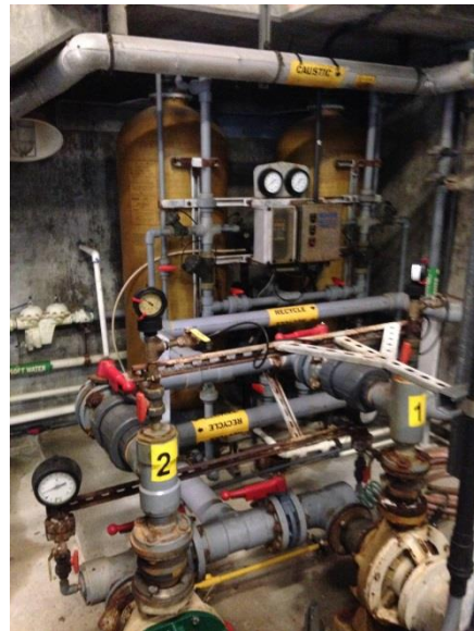
Chemical Piping and Water Softening Tanks
