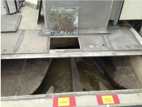
Influent Junction Chamber
