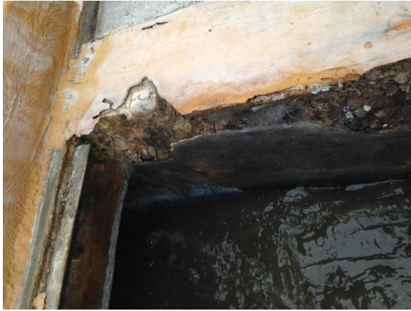
Grit Influent Channel
