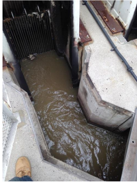
Screenings Influent Channel
