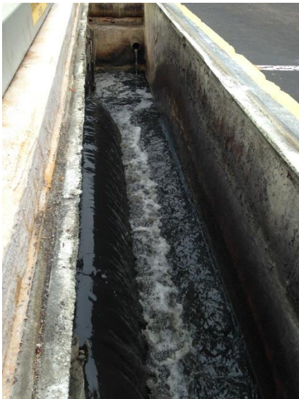
Grit Effluent Weir and Channel
