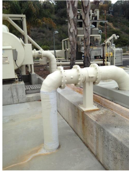
Odor Control Duct Corrosion
