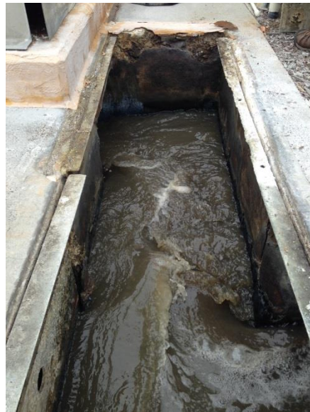
Grit Influent Channel
