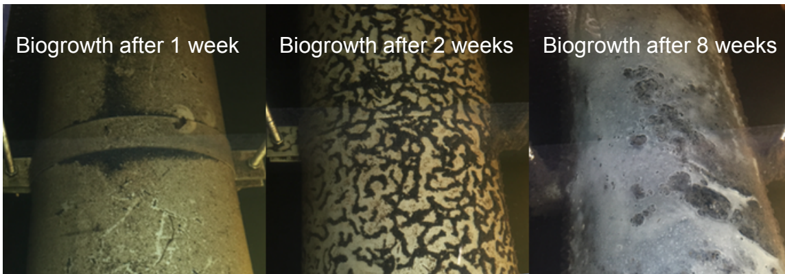
Figure 8 – Biogrowth observed on filtrate pipes from three Dynasand filters at the SEWRF: Filter 3 after 1 week of operation (left), Filter 2 after 2 weeks of operation (center), Filter 1 after 8 weeks of operation (right)
