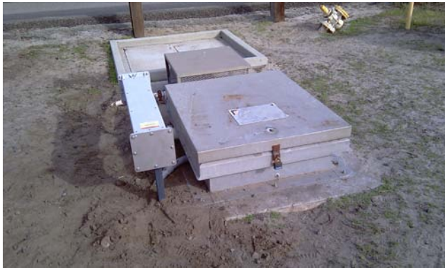
Coast Pump Station showing completed electrical upgrades.
