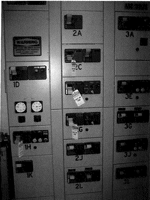
MCC-B is one of several electrical assets nearing the end of their useful lives that will be evaluated.
