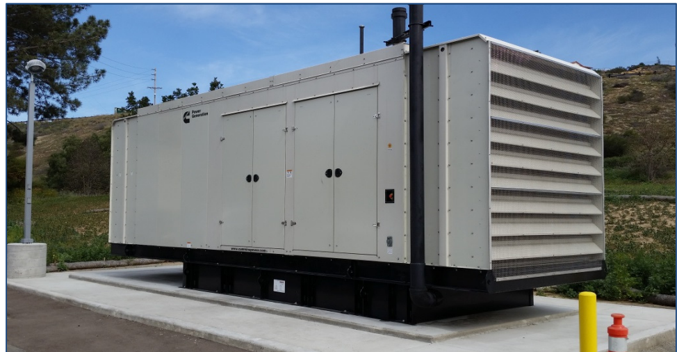
SEWRF Emergency 800 kW Generator
