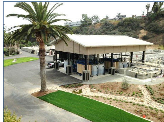
Advanced Water Treatment Facility
